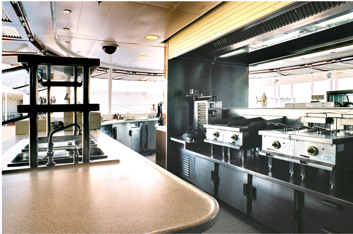
Outside bar showing a pair of table top griddles and table top fryers built in stainless steel 316L
